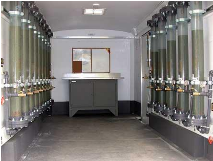
A self-contained, mobile system, the pilot unit typically consists of four to eight four-inch-diameter columns measuring four vertical feet. The number of columns may vary depending on the radium concentration in the water and the length of the pilot test.
