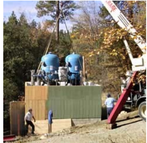
Water company officials say residents and tourist at Bass Lake no longer need to worry about uranium in their taps and faucets. The uranium treatment facility was designed and constructed by Water Remediation Technologies.
