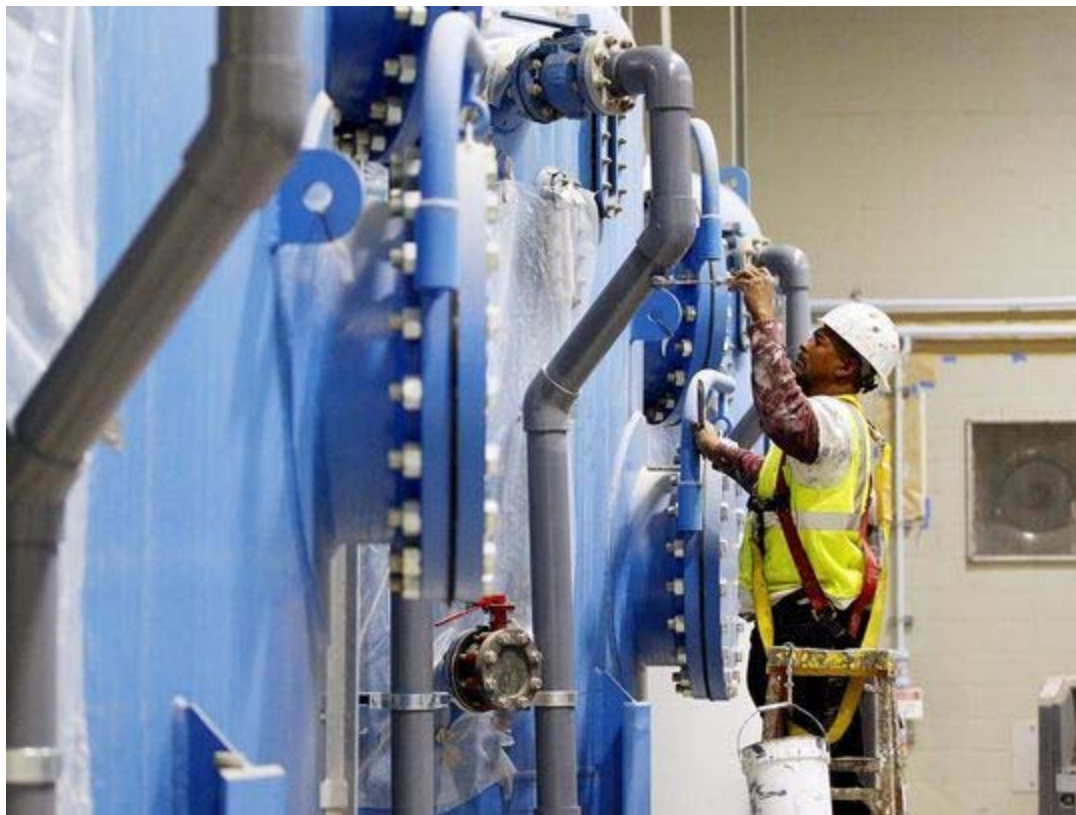
Brady will use filtration tanks similar to the ones at San Angelo's water treatment plant. (Photo: Standard-Times file)
