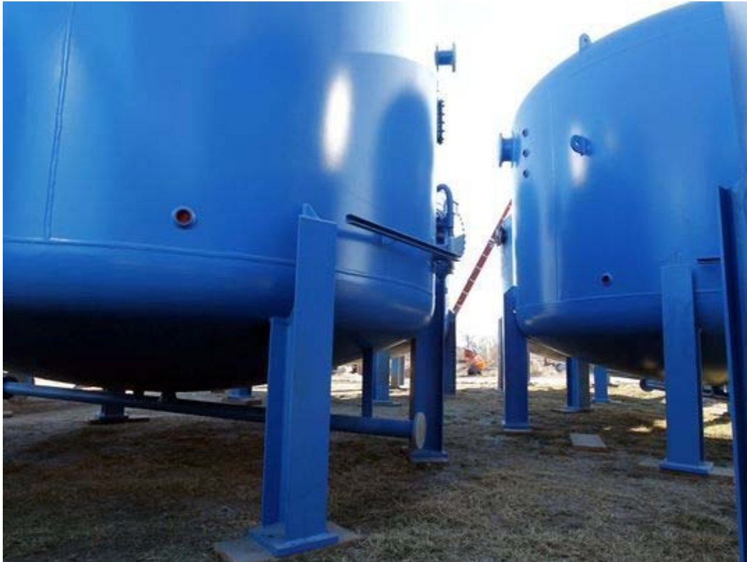
Water filtration tanks wait to be placed in the groundwater treatment plant in San Angelo in 2014. Brady will use a similar filtration system to San Angelo's to help reduce the amount of radium in water from the Hickory Aquifer. (Photo: Standard-Times file)
