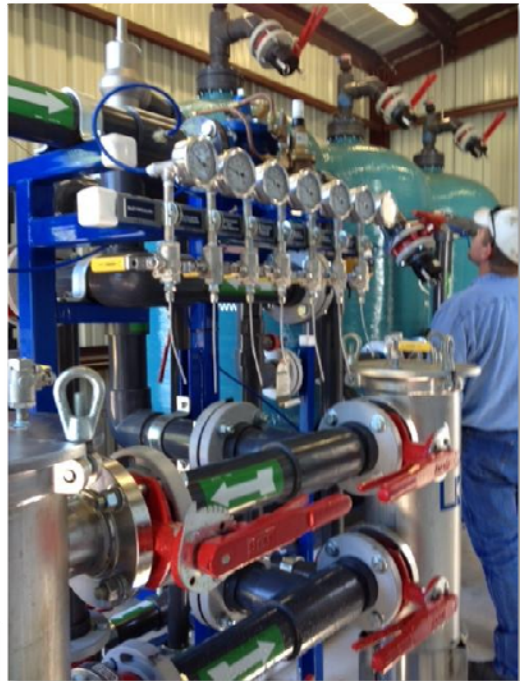
Face piping and sampling station
