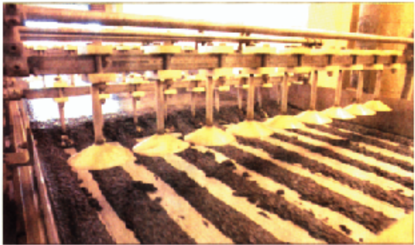
Waste water sludge is processed at the Batavia Water Treatment Plant before being sent to a landfill.
