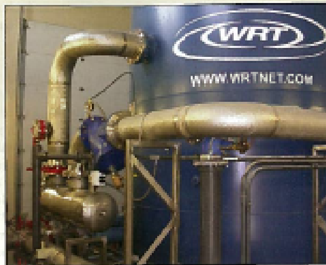
Water Remediation Technology has installed two radium removal systems for the village of Antioch, Ill., and is responsible for removal of the spent treatment media to a licensed disposal facility.
